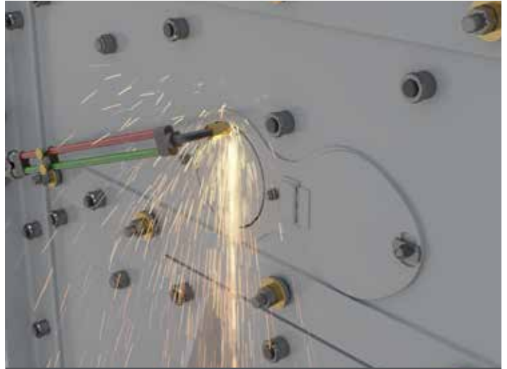
02/ SPRAY BAR KNOCKOUTS
