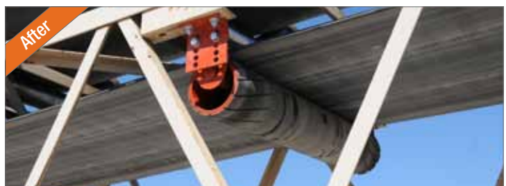
Belt Straightened Immediately After Installation
